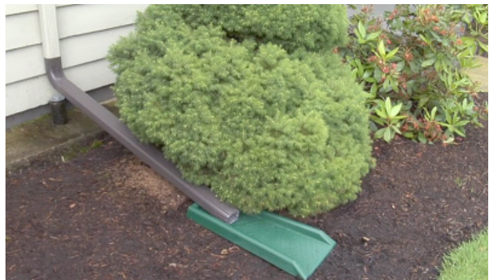
Downspout disconnection as part of the Cornerstone Projects. Credit: City of Portland
